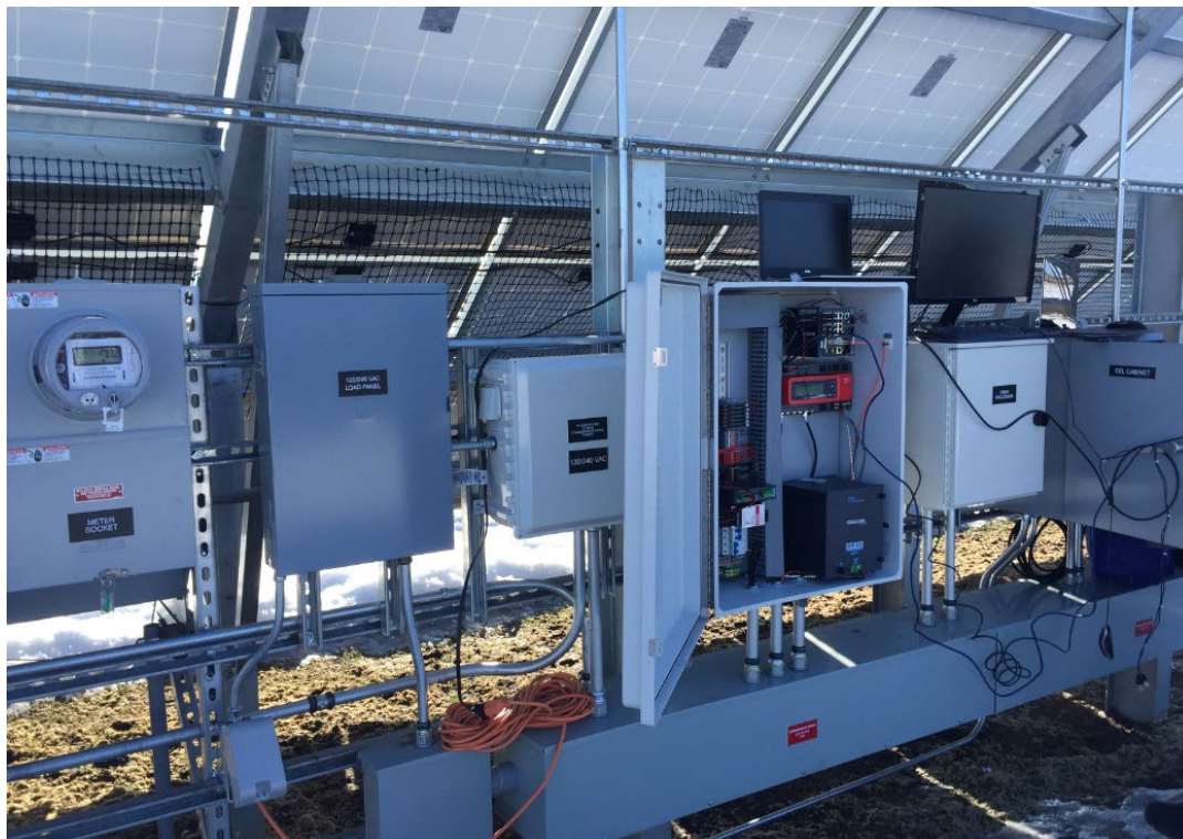
Figure 8-5. Bozeman Solar Microgrid Container Boxes and Controllers
