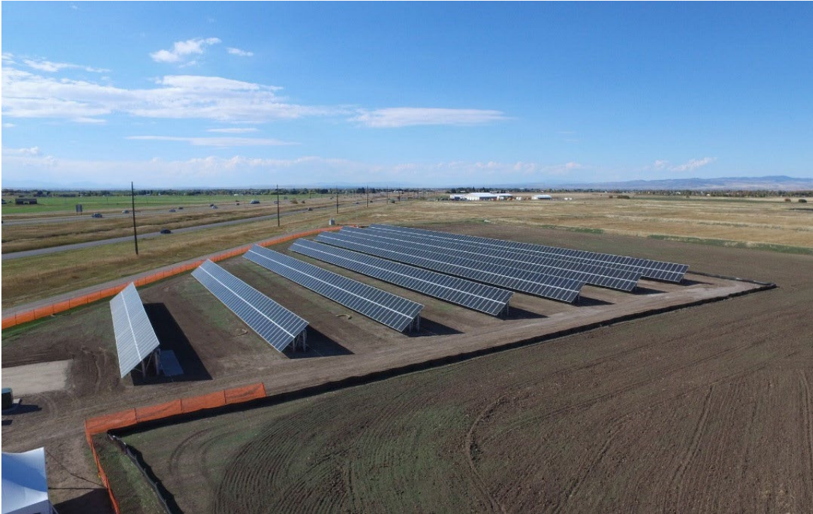
Figure 8-6. Bozeman Solar Microgrid 380 kilowatt Array
