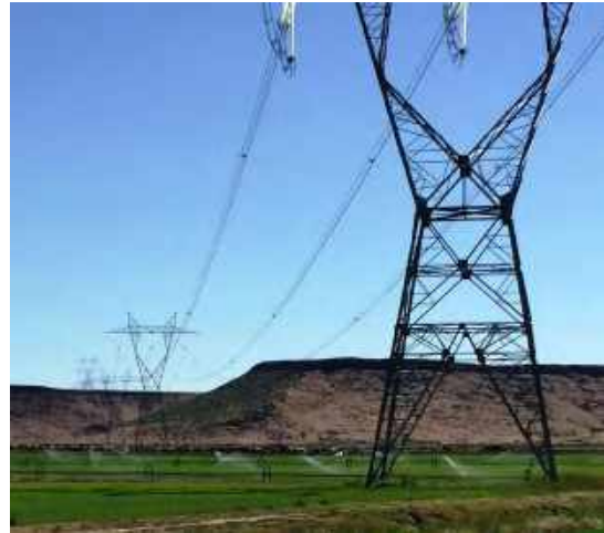
500-kilovolt (kV) transmission line near Melba, Idaho
